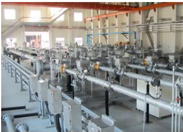
Figure 4: CPC large capacity re-circulation flow system.
