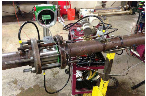
Fig 8. The Prototype Mass Meter Installed at CEESI.
