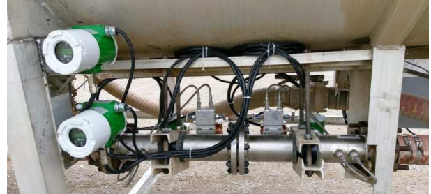
Fig 23. Front View of Meter Installations.
