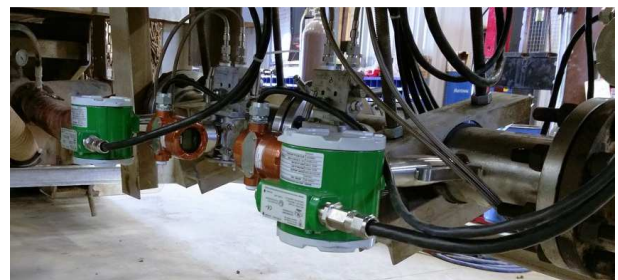
Fig 24. Back View of Meter Installations.
